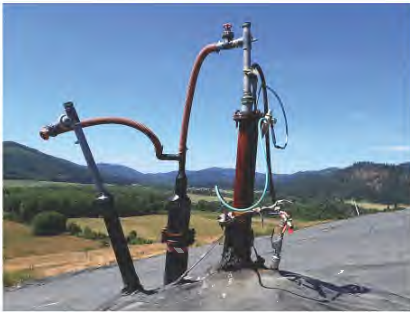
Gas well 3V81, flagged by the EPA for leaking landfill gas, June 2024. The liner has pulled away from the support on the left and landfill gas is coming out at over 14,000 ppmv, over 28 times the actionable limit.
